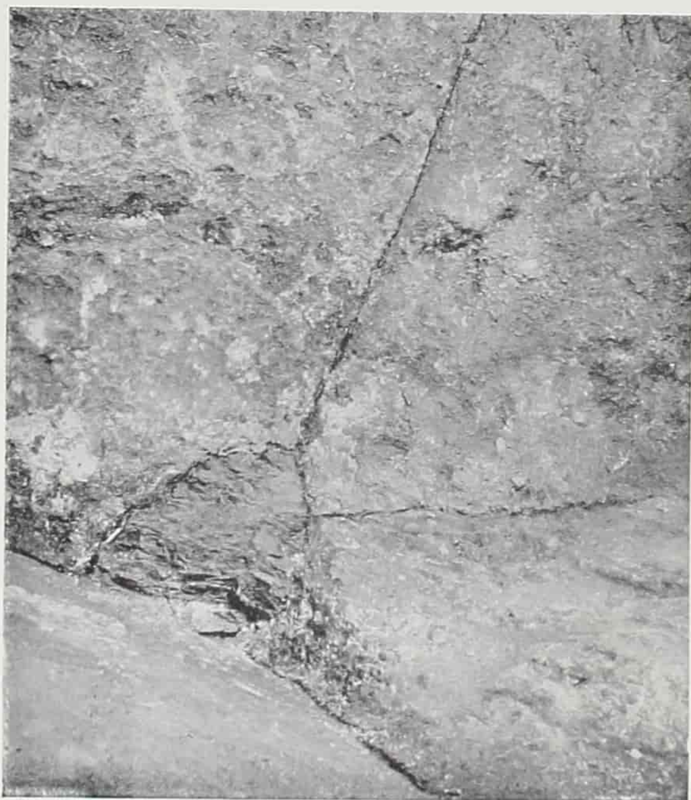
The bottom east corner at the lower end of the Descending Passage of the Great Pyramid of Gizeh, showing the hard natural concrete filling the corner.
