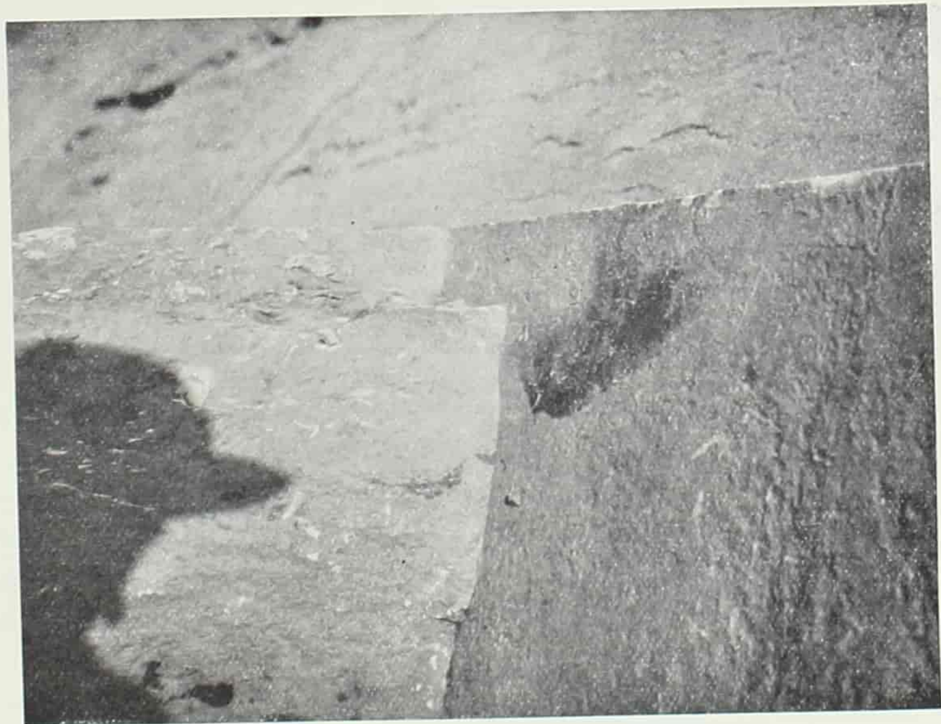
A fractured butt-joint between the pavement (on the left), and the bevelled front edge of the platform (on the right) in front of the casing-stones of the Great Pyramid of Gizeh.
